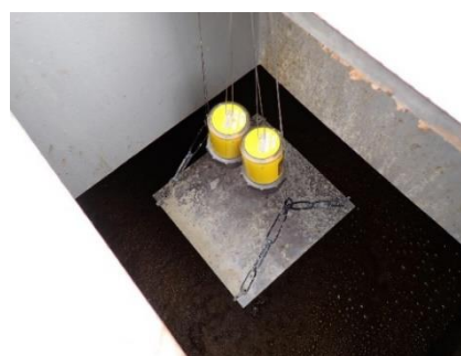
Fig.2 硫化水素濃度測定器設置状況 Installation Status of Hydrogen Sulfide Measuring Device
